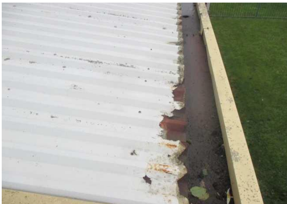
Corroded Edges to Cladding
